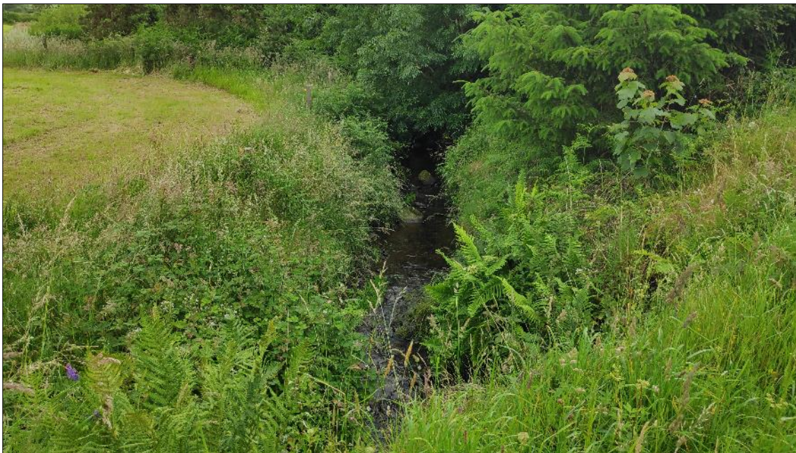
Plate 8B.4-33: Representative image of site C17 the Coolaniddane River (upstream of road culvert)
